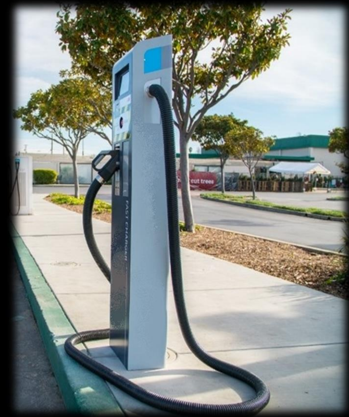
Mode 4: Simulating the Connection to a DC Charging Station.
